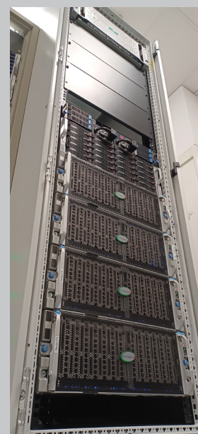
The new server rack includes four BetaBufs, one FlexBuff, and a GPU server above them.
